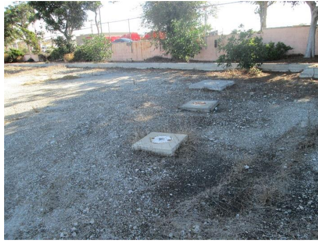
14. Typical groundwater monitoring wells.
